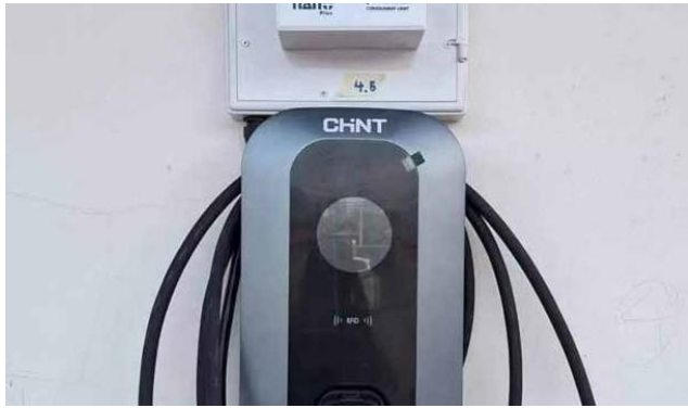
22kW AC Charger Private home EV charger, Thailand
